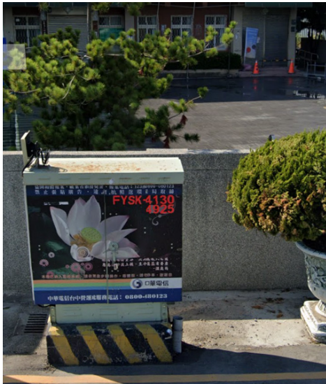
Figure 15. Chunghwa Telecom's cross-connect cabinet
