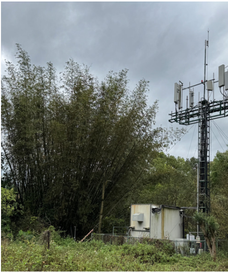
Figure 12. Chunghwa Telecom's base station
