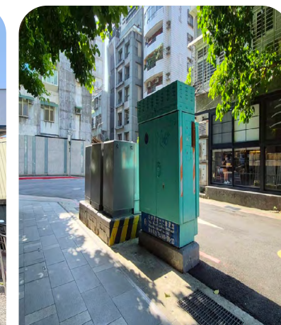
Figure 14. Chunghwa Telecom's cross-connect cabinet
