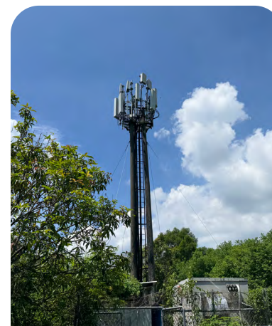
Figure 11. Chunghwa Telecom's base station
