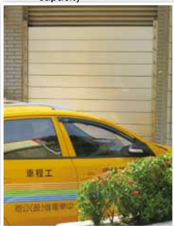
Water resistant panels installed in lowlying area equipment rooms to ensure communications during rainstorms.
