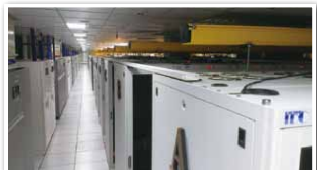
With the rise of the cloud service, we bolster energy saving at datacenters to achieve green ICT.
