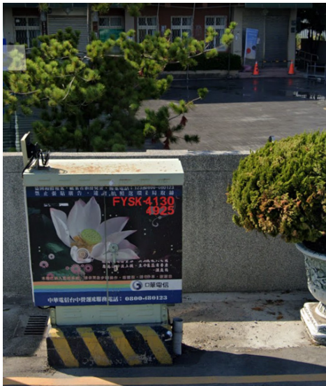
Figure 15. Chunghwa Telecom's cross-connect cabinet
