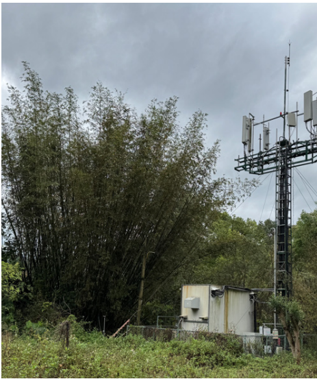
Figure 12. Chunghwa Telecom's base station
