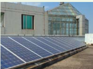
We installed photovoltaic panelplates at appropriate locations to save the cost of electricity.
