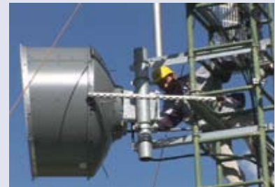
Undertook microwave construction projects in rural areas to provide telephone and Internet connection services.
